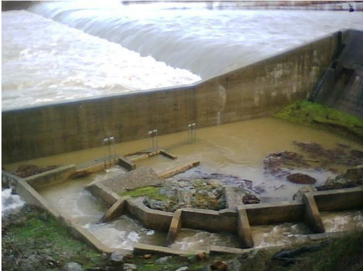
Figure II-c. South fish ladders at Daguerre Point Dam during high flow conditions (YCWA 2010).
