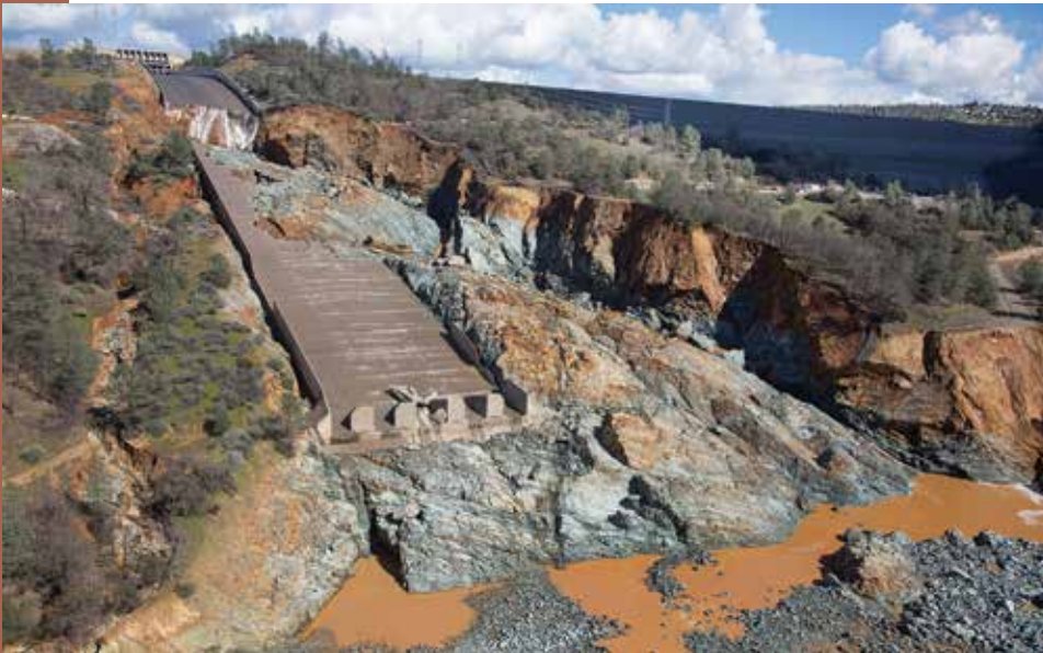
Oroville Dam Spillway, Feb. 27, 2017. The Oroville dam main spillway after spill flow releases ceased for repair inspections. Oroville Dam is in the shadow on the upper right. Source: Dale Kolke, CA Dept. of Water Resources (hereby DWR).
