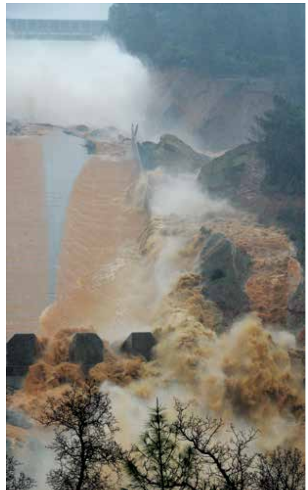
Damaged Oroville Main Spillway. Mud and debris tumble down the newly eroded channel alongside the Oroville main spillway on Feb. 8, 2017. Source: Bill Husa, Chico Enterprise-Record.
