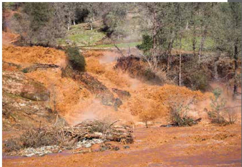
Oroville Dam Spillway Erosion, Feb. 11, 2017. Water and debris from the emergency spillway failure flow into the diversion pool just downstream of the dam. Source: Dale Kolke, DWR.
